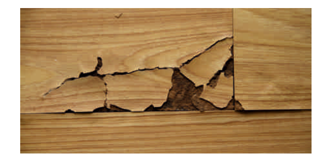
No claim will be entertained For cracking arising our of Groove currying or l. Shape
