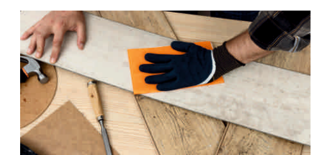
Extra care required in vertical pasting of laminated Sheet as there is possibility of bubbles due To lack of uniform pressure.
