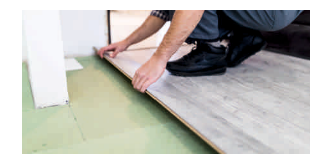
Cracking at corners & around cuts may be caused By improper conditioning, improper bonding, poor planning. Avoid all these to prevent cracking at corners.
